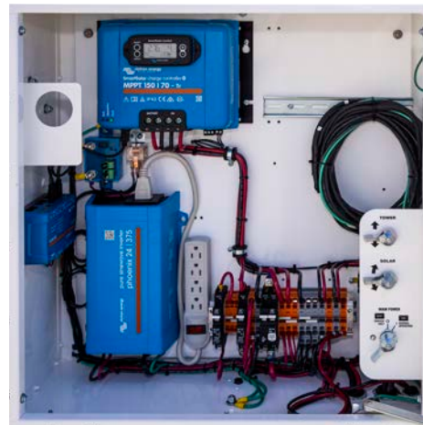
Control box wired and ready for installing electronics
